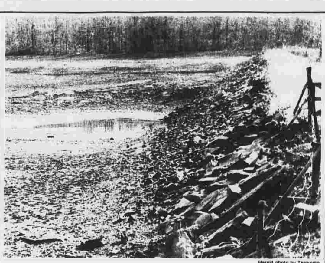
The Risley reservoir on Lake Street, once a scenic area, has become a mere puddle because of a dam that needs repairs. But the repairs appear a long way off because no one wants responsibility for the problem.
